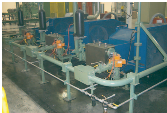
Pump Unloading/Relief Manifolds
